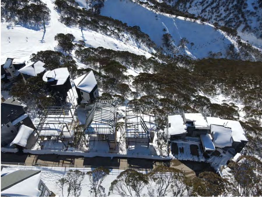
Figure 3.4: Subject land looking north east
