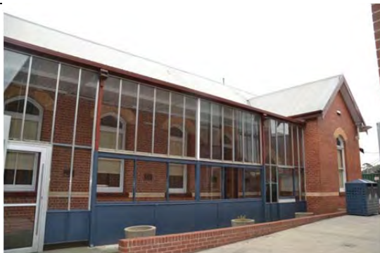
Pell Wing (old Science Wing), north elevation (east portion), March 2014, showing introduced glazed verandah.
