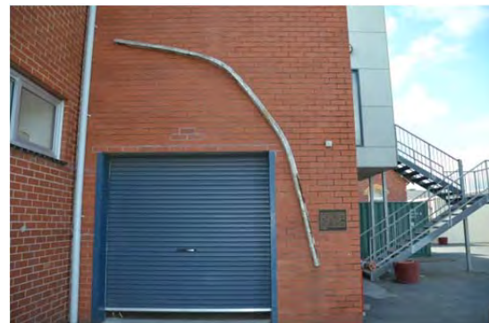
Miller Wing, west elevation, showing remnant iron mine shaft rail attached to wall, 2014.
