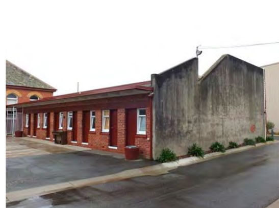
Change Rooms, west and south elevations, showing rendered original hand ball wall, 2014.
