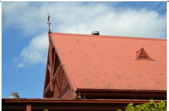
Whelan Food Centre (former dining hall), detail of north gable end looking east, March 2014.
