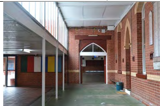
Verandah/covered way of Pell Wing, west elevation north end. Note the brick wall with pointed-arched opening built in 1909 and shown in the historical photograph of 1916-17 (left in foreground), March 2014.
