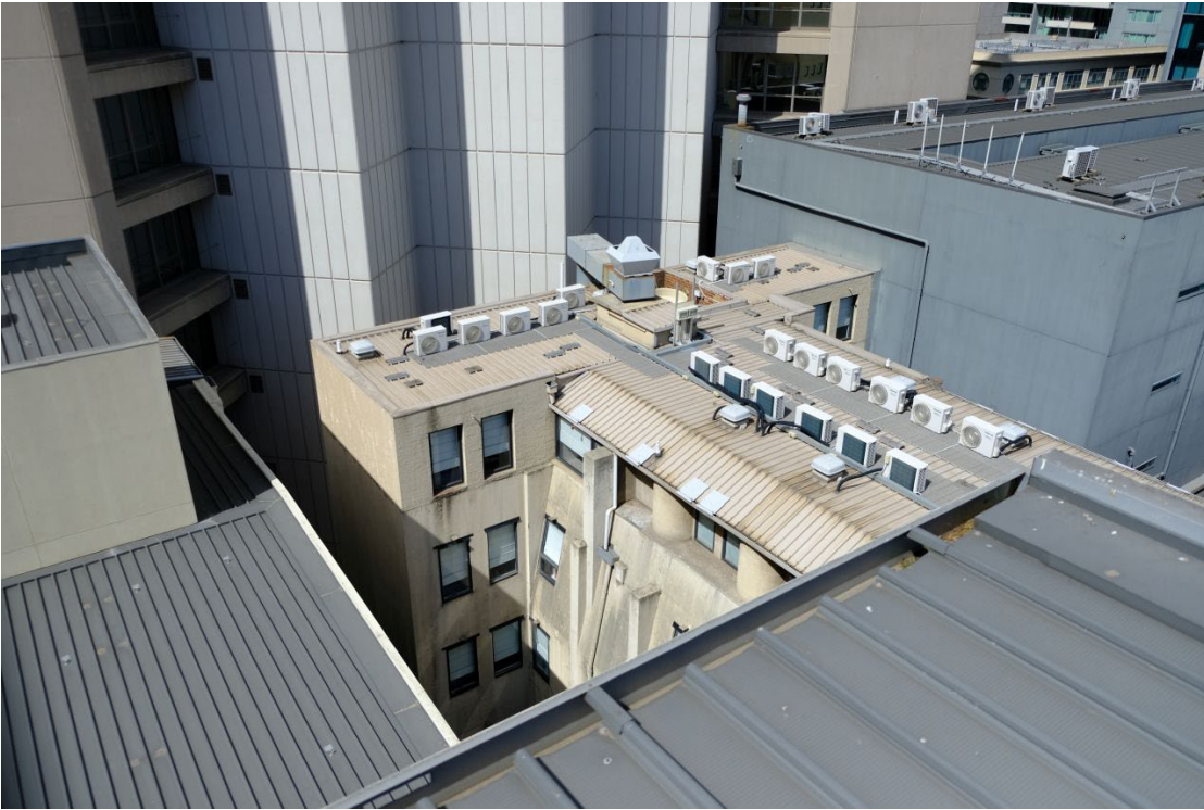
Figure 23 Later roof and fifth floor level addition viewed from the roof of the State Savings Bank
