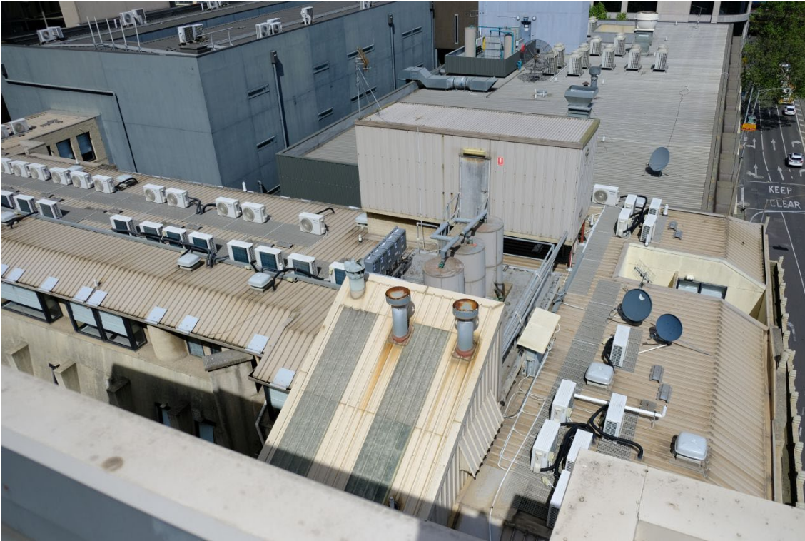
Figure 34 The roof of the Batman's Hill Hotel showing the modern mansard roof to the added fifth level.
