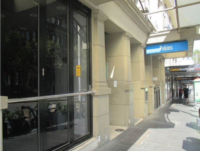
Figure 36 Later alterations to the street level Collins Street elevation including enlarged openings, inset door, modern windows and doors, glazed arched awning and re-rendered façade
