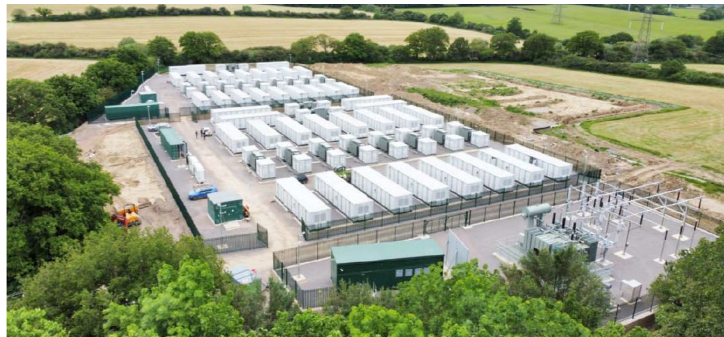
Figure 2-2 Typical Bess Layout
