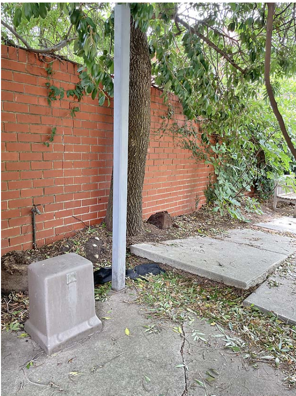
Image 15: Shows the base of Tree 37 with the uplift of concrete pavement and location of services.
