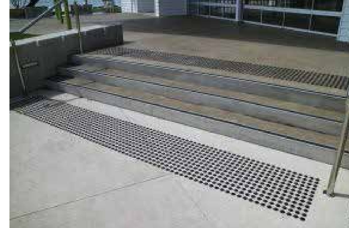
All insitu concrete steps to include DDA compliant TGSIs, nosing & stainless steel handrails
