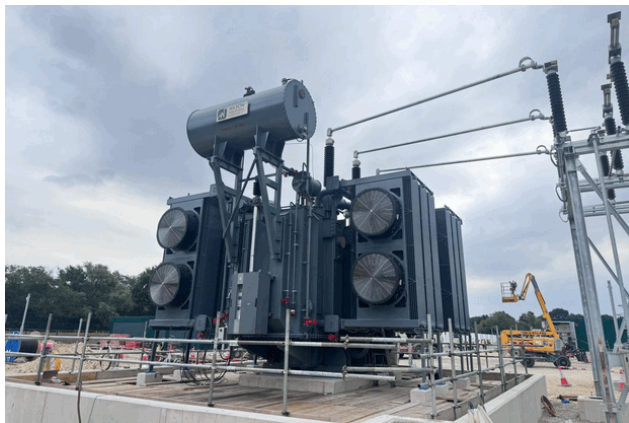
Figure 6 Photo of transformer
