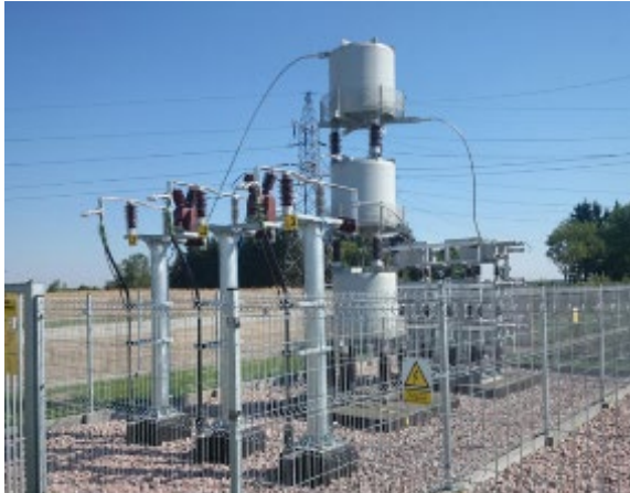
Figure 7 Photo of Harmonic Filter
