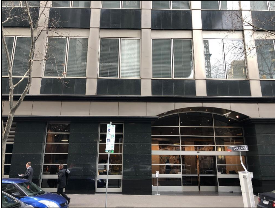
Figure 9 Image showing the west elevation of the RBA building to Exhibition Street. The non-original segmented stainless steel cladding to the columns of the upper levels, granite clad piers and infill glazing of the ground floor level are apparent.
