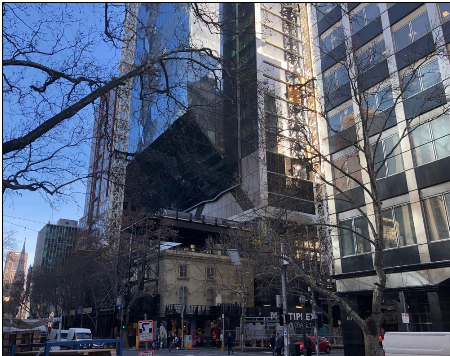
Figure 12 View toward the registered building at 68-72 Collins Street with the redevelopment of 80 Collins Street under construction. The subject site is to the right.
