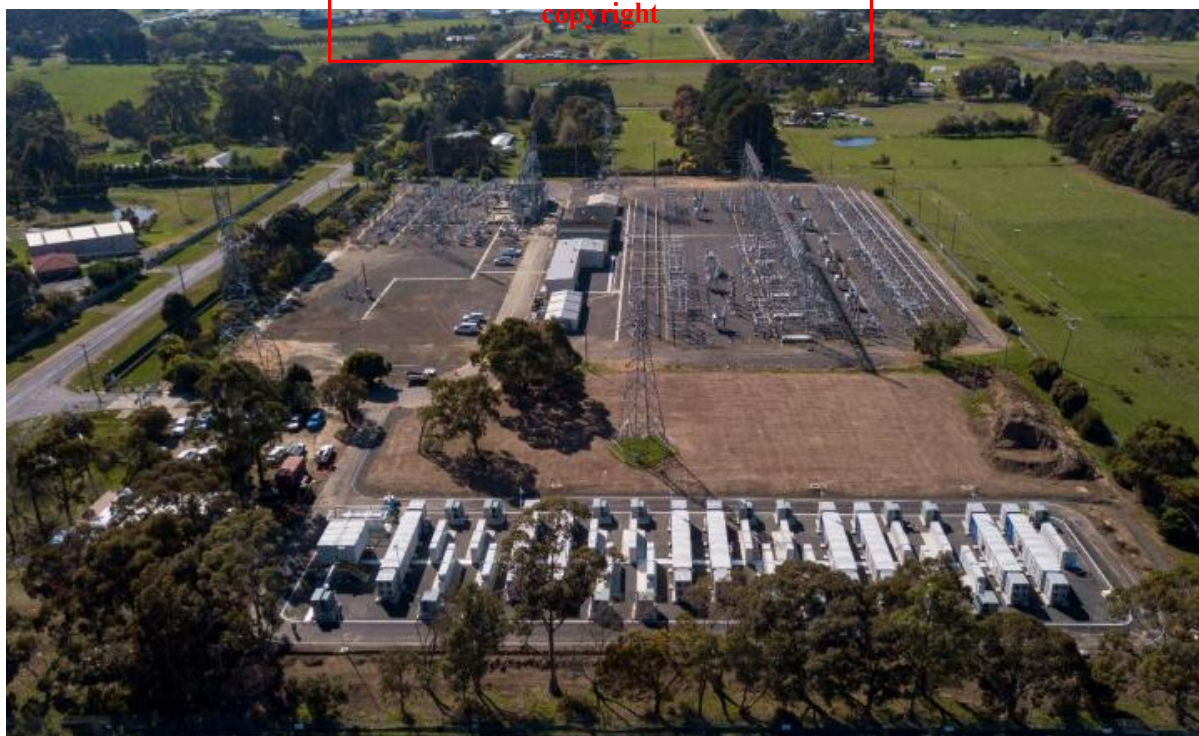
Figure 11 Example BESS Installation
