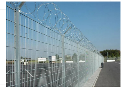
2.4m High Substation security fence
