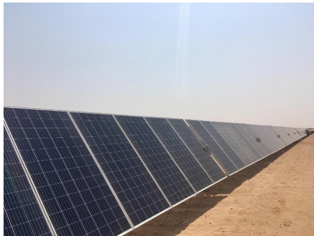
Mounted single-axis bifacial tilting panels.
