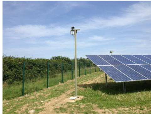
Picture 4 Example CCTV Cameras
