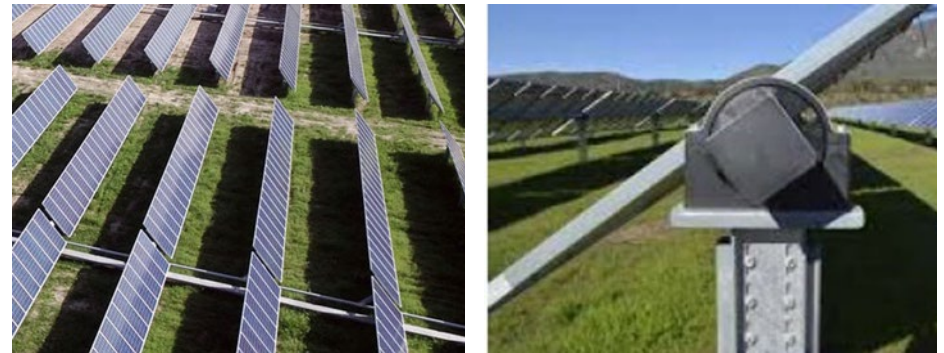
Picture 1 Typical Mounted Panels (single axis tracker)
