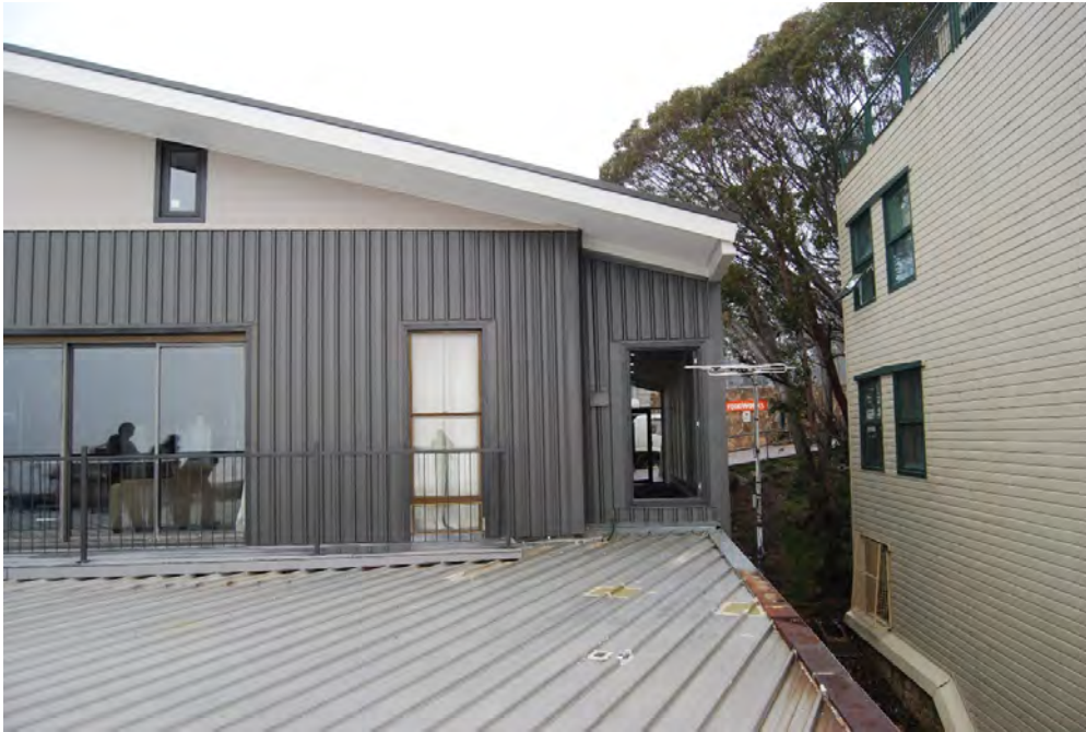
Figure 5: View of main works zone. On top of Level 1 roof. Edges to have fall-barrier installed for works. Roof access point from common hallway shown.
