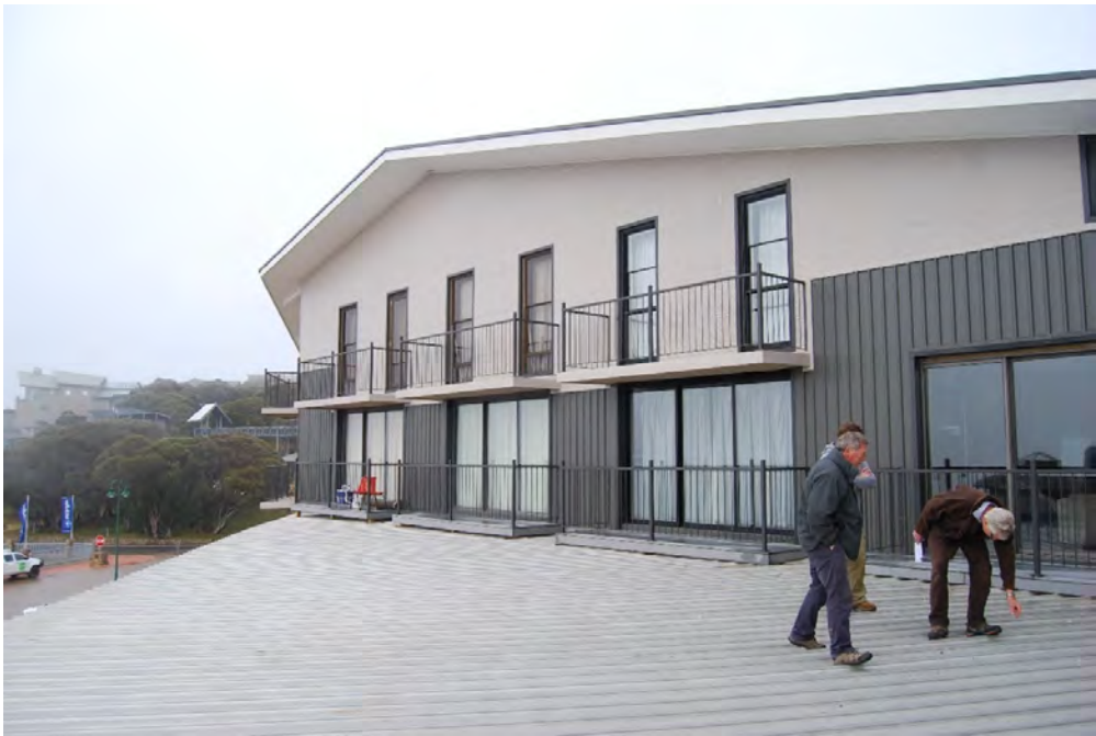
Figure 4: View of main works zone. On top of Level 1 roof. Edges to have fall-barrier installed for works.
