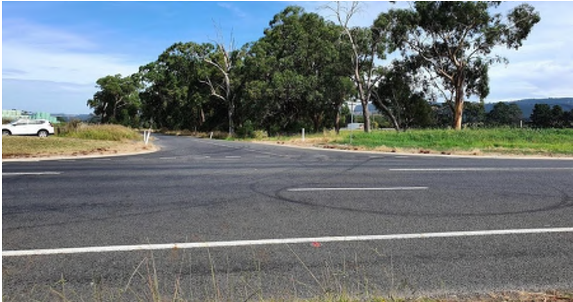
Figure 5 Green Gully Road – priority intersection with Strzelecki Highway (Source: AECOM photo taken 19/03/2020)
