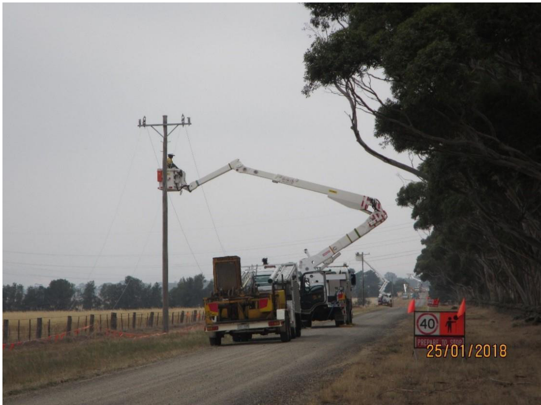
Figure 5: Example of contractors working on the new or replacement installation. Note the truck is still in the road carriageway.
