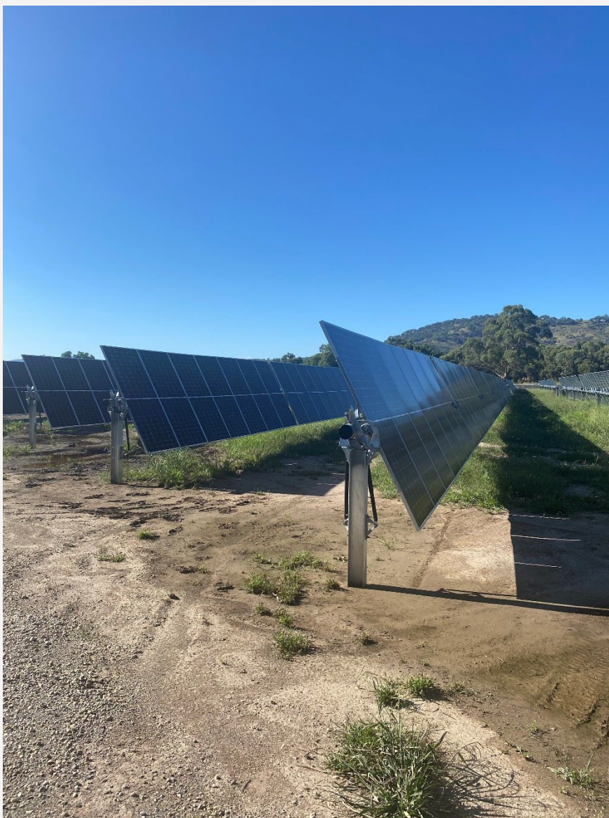
Figure 15 – Example of a single axis tracker system in a single portrait orientation. The example shows the panels at full 60-degree tilt.
