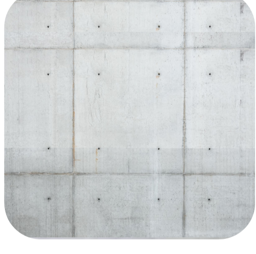
OFF FORM CONCRETE
