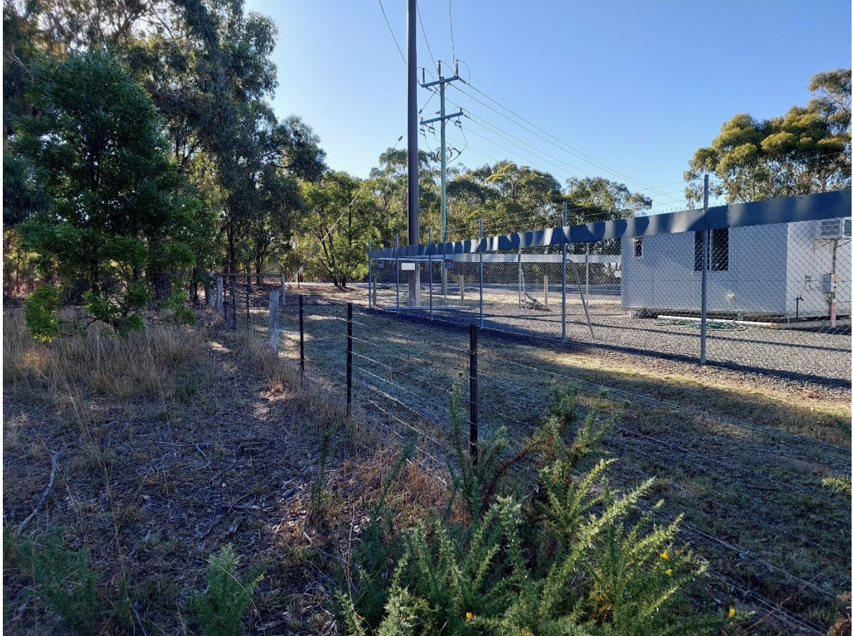
Photo 5. Gisborne Substation on the eastern edge of the Project Area
