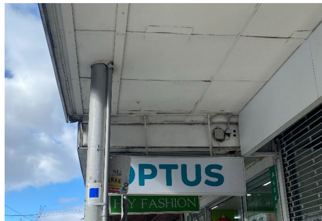
Figure 3-25. Overhead pole through the awning at 143-145 Hopkins Street, facing east
