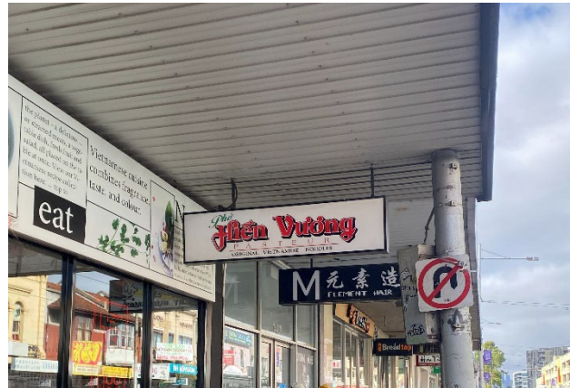
Figure 3-23. Overhead pole through the awning at 144 Hopkins Street, facing east
