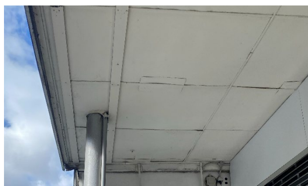
Figure 4-6. Overhead pole through the awning at 143-145 Hopkins Street, facing east
