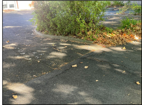
Image 2. Significant heaving of asphalt indicating surface roots from Tree 28.
