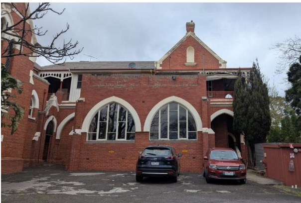
Figure 12 Northern elevation of c.1889 main building showing the intrusive 1963 enclosing the ground floor verandah
