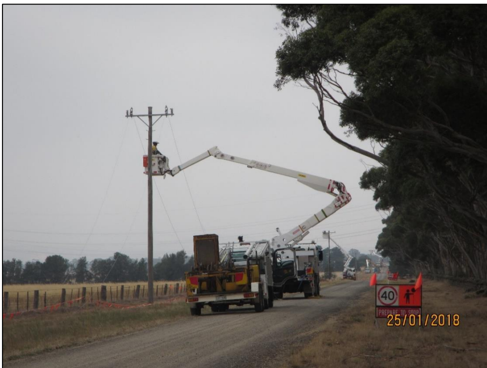
Photograph 4 – Example of contractors working on a new or replacement installation (note the truck is still in the road carriageway)
