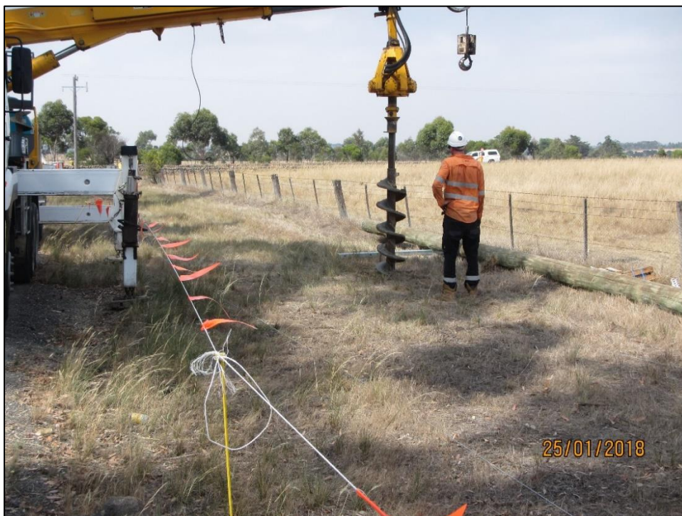
Photograph 2 – Example of a hole being augured via an arm from truck (note in this example the roadside vegetation was deemed to be native in places and fencing was erected to prevent the truck from entering the road shoulder)
