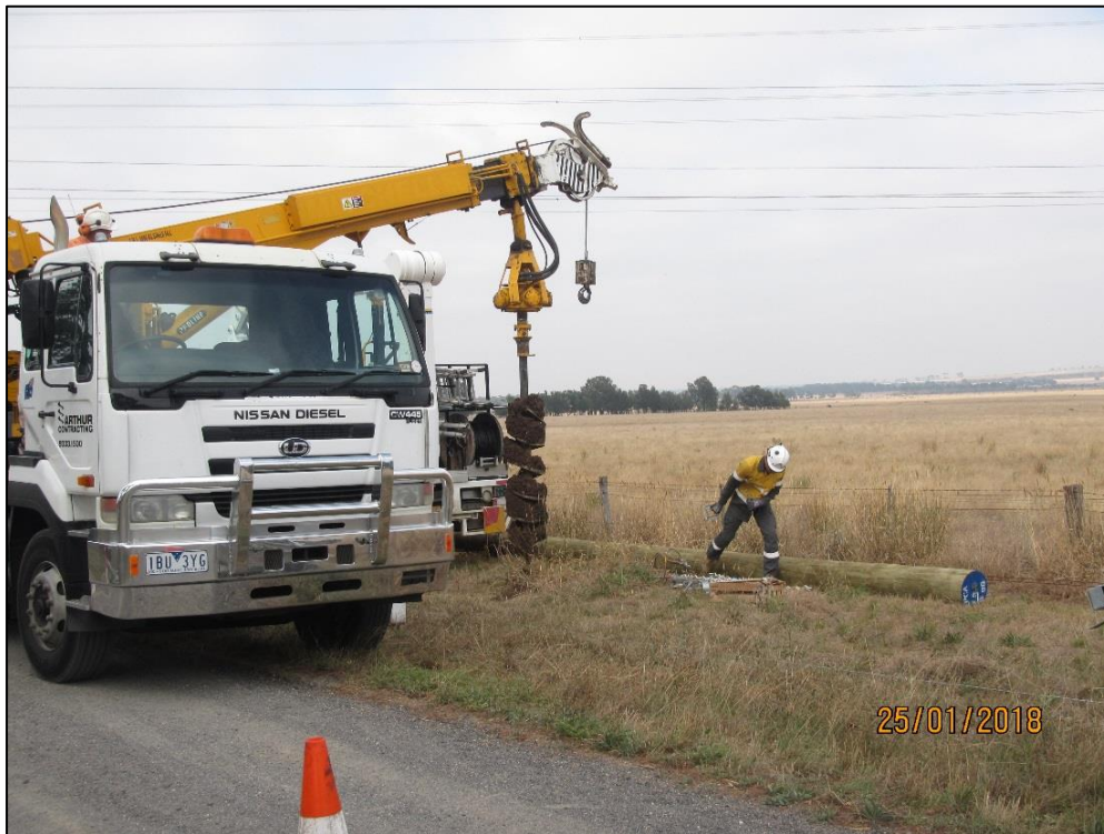
Photograph 1 – Example of a hole being augured via an arm from truck (note in this example the roadside vegetation was deemed to be non-native, hence the truck parking slightly on the verge and the other truck in the background)
