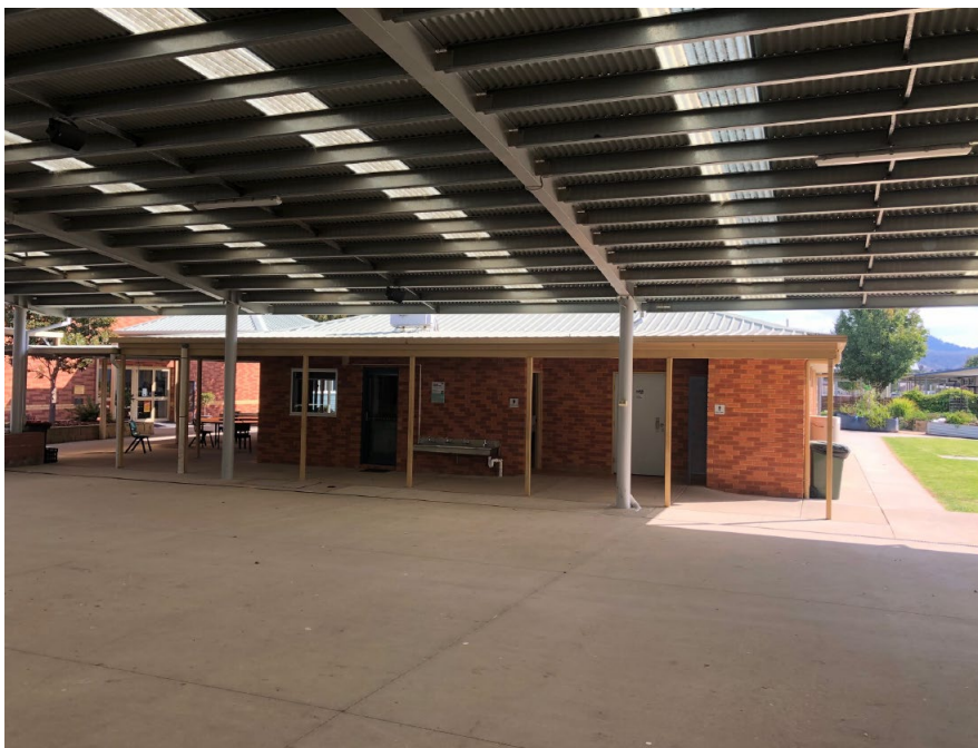
Figure 6 View of existing Hudson building to be demolished from the covered outdoor learning area (Source: Permit application)
