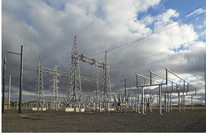
Figure 6 – Typical Terminal Station.
