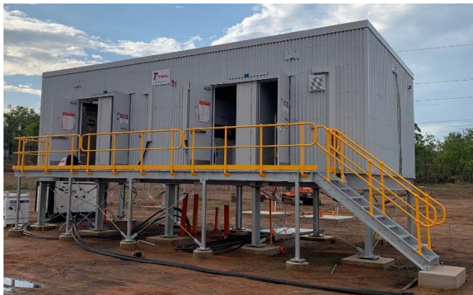
Figure 7 – Typical HV switchgear room – rear elevation (Source: T2 Energy).
