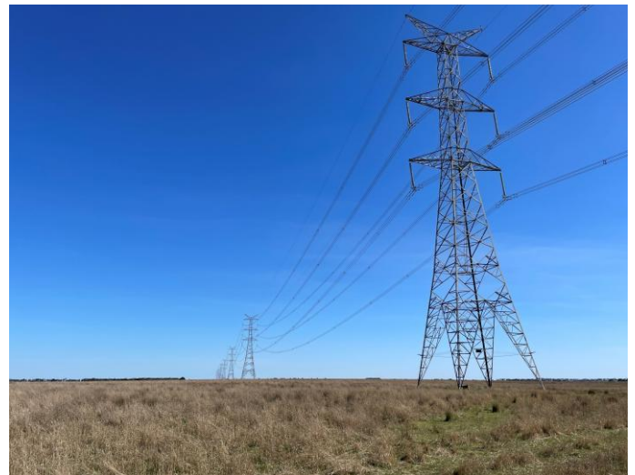
Figure 6: Existing 500kV Moorabool to Mortlake powerline that bisects the project area, viewed from Darlington-Terang Rd.
