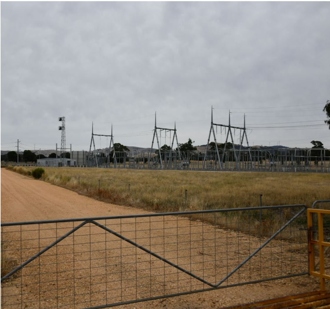
Figure 3-3 On-site substation example
