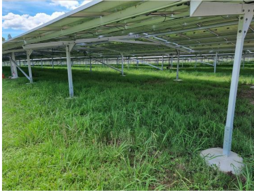
Figure 23. Image from Birdwood Energy showing the SMS system installed.
