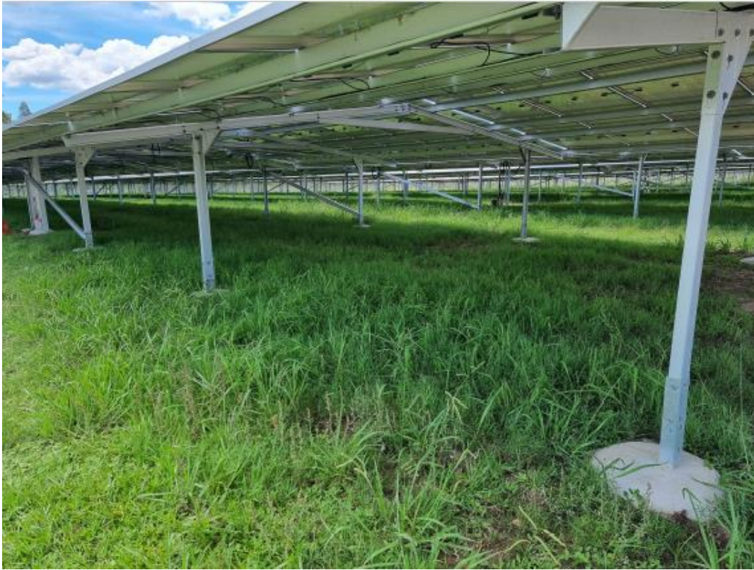
Image 6: A recently constructed PV array using the SMS east-west system.
