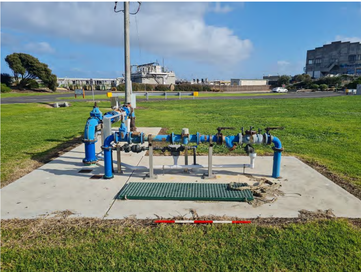
Plate 34 Water Infrastructure facing west (R. Stewart 11.07.2023)
