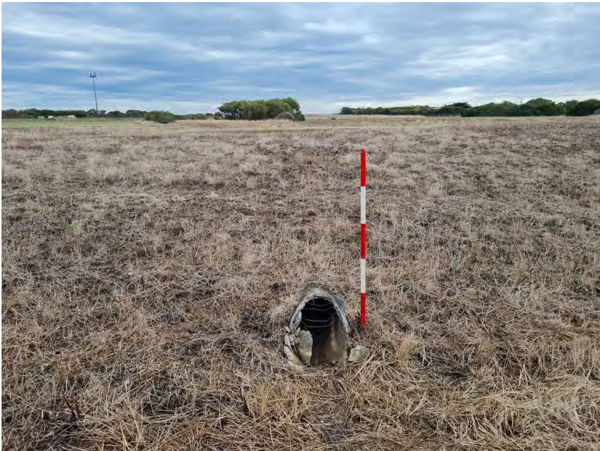
Plate 72 Overflow drain in dam wall, southeast corner of dam, facing west (R. Stewart 26.04.2023)
