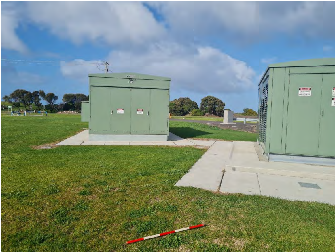
Plate 31 Substation facing south, with drainage and water infrastructure in the background (R. Stewart 11.07.2023)
