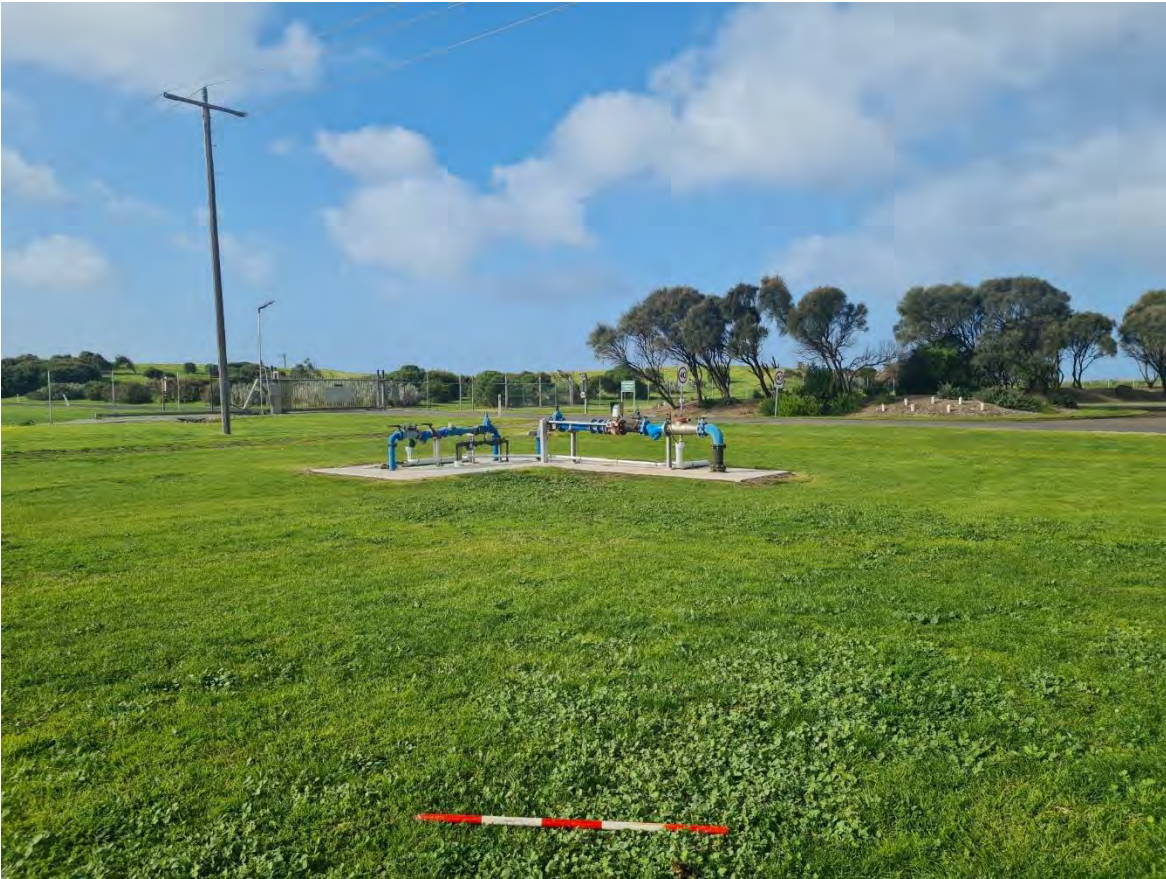
Plate 33 Facing southeast towards entrance gate, with water infrastructure in the foreground (R. Stewart 11.07.2023)
