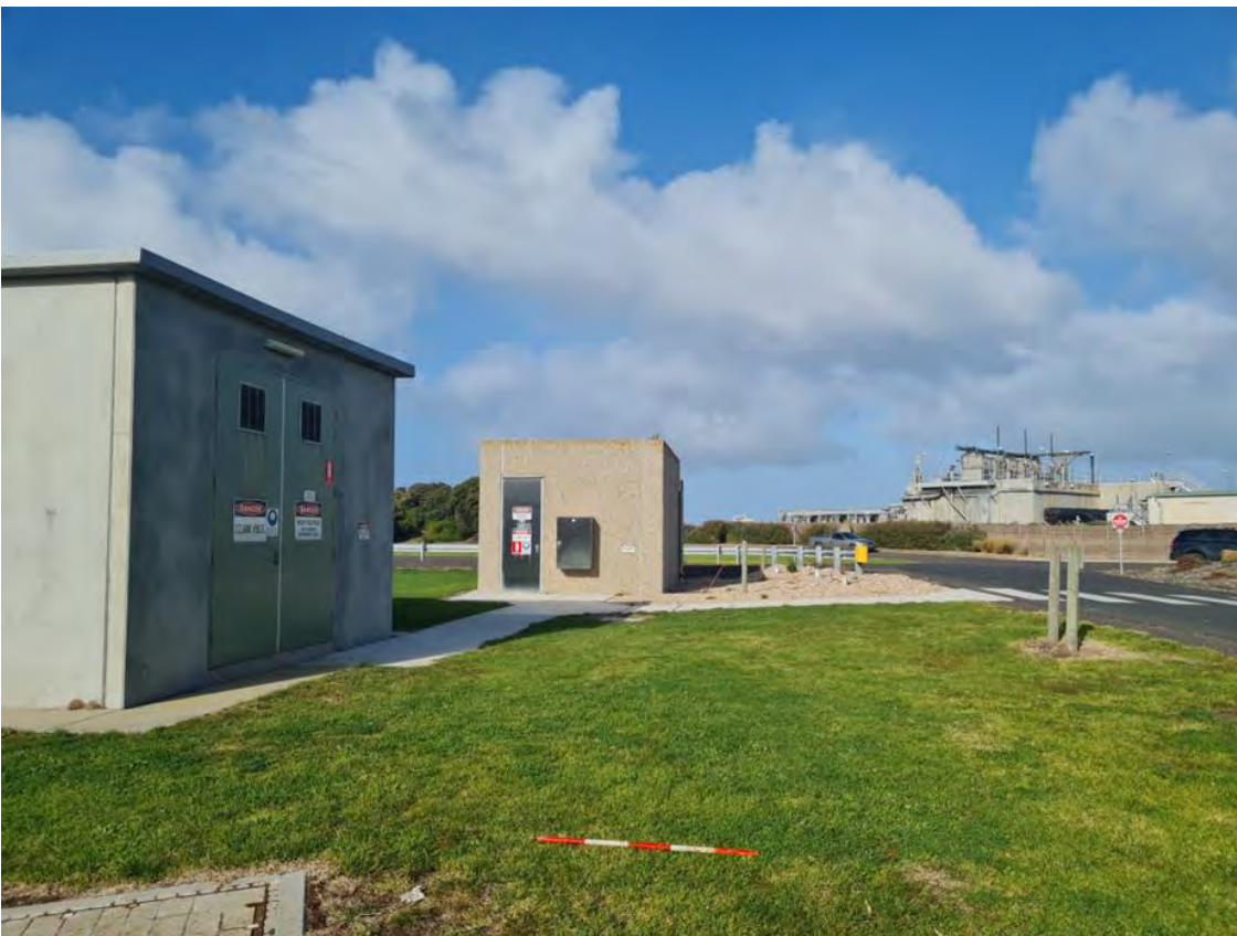
Plate 30 Substation in west, facing south (R. Stewart 11.07.2023)
