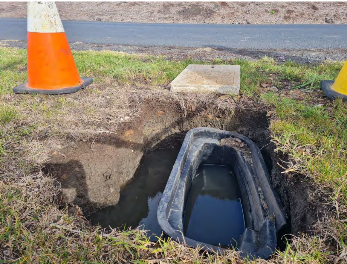
Plate 42 Open utility pit in west of Activity Area – Upper context of reddish brown likely fill, lower grey-black consistent with natural soil profile (see geotechnical logs) (R. Stewart 11.07.2023)
