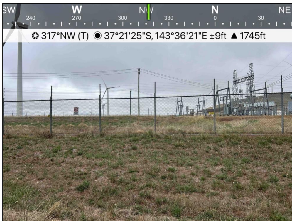
Figure 8 – Managed grass around the Waubra Terminal Station.
