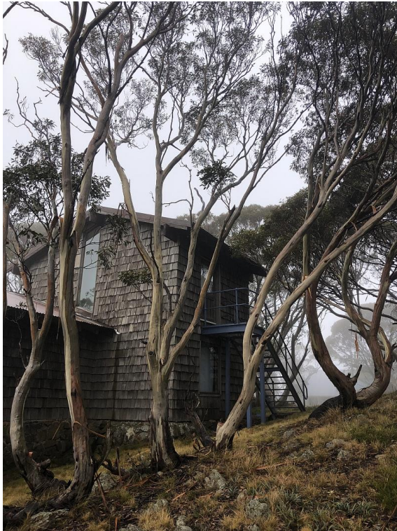
Plate 1 Photo is looking toward the north west corner of the existing building
