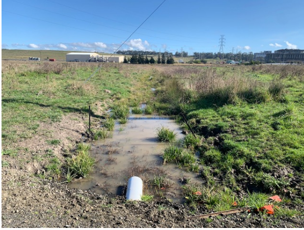
Figure 2-5: Drainage channel extending from MWTS – view west
