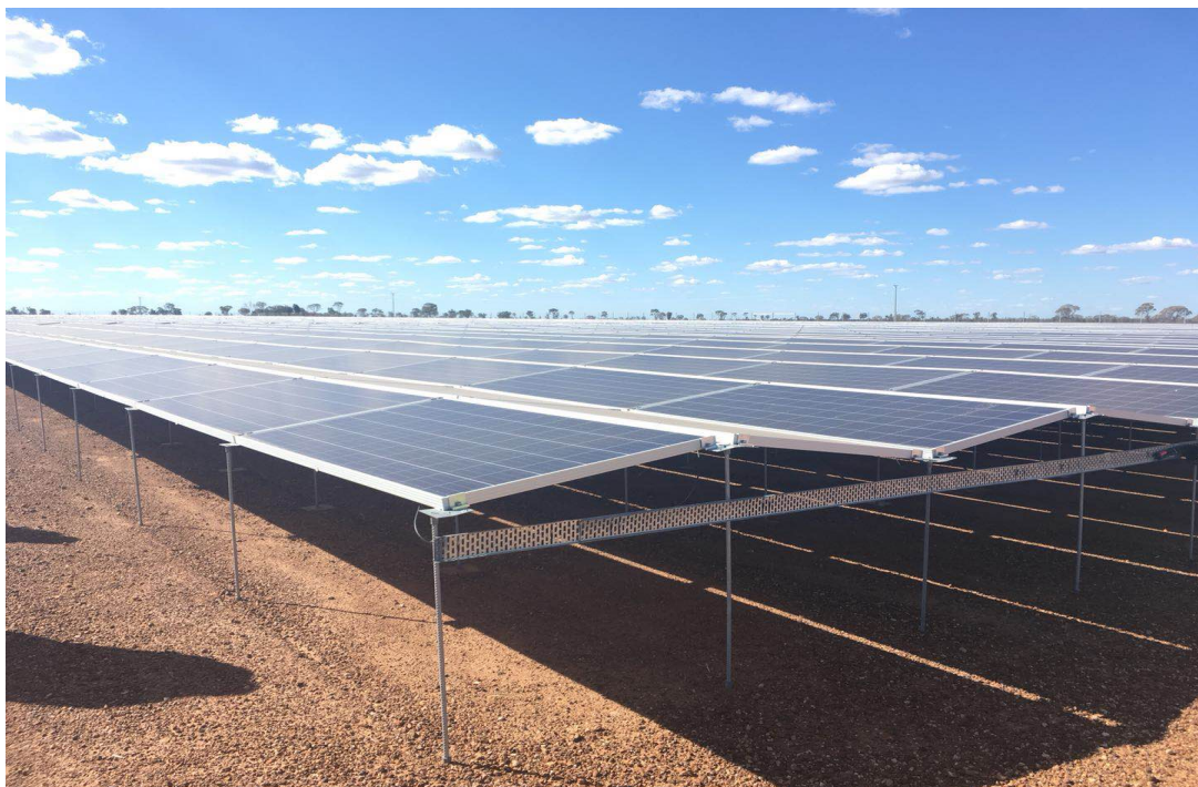
Figure 5. Typical PEG Solar Panels
