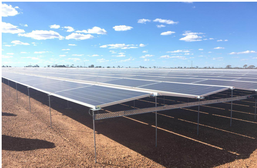
Figure 5. Typical PEG Solar Panels
