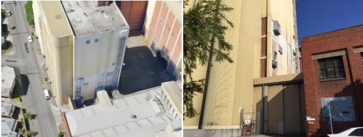
Figure 5: North face of the site showing suspected flour dust emitted on wall. Google Maps accessed 15/5/17. Photograph taken 16/5/17.
