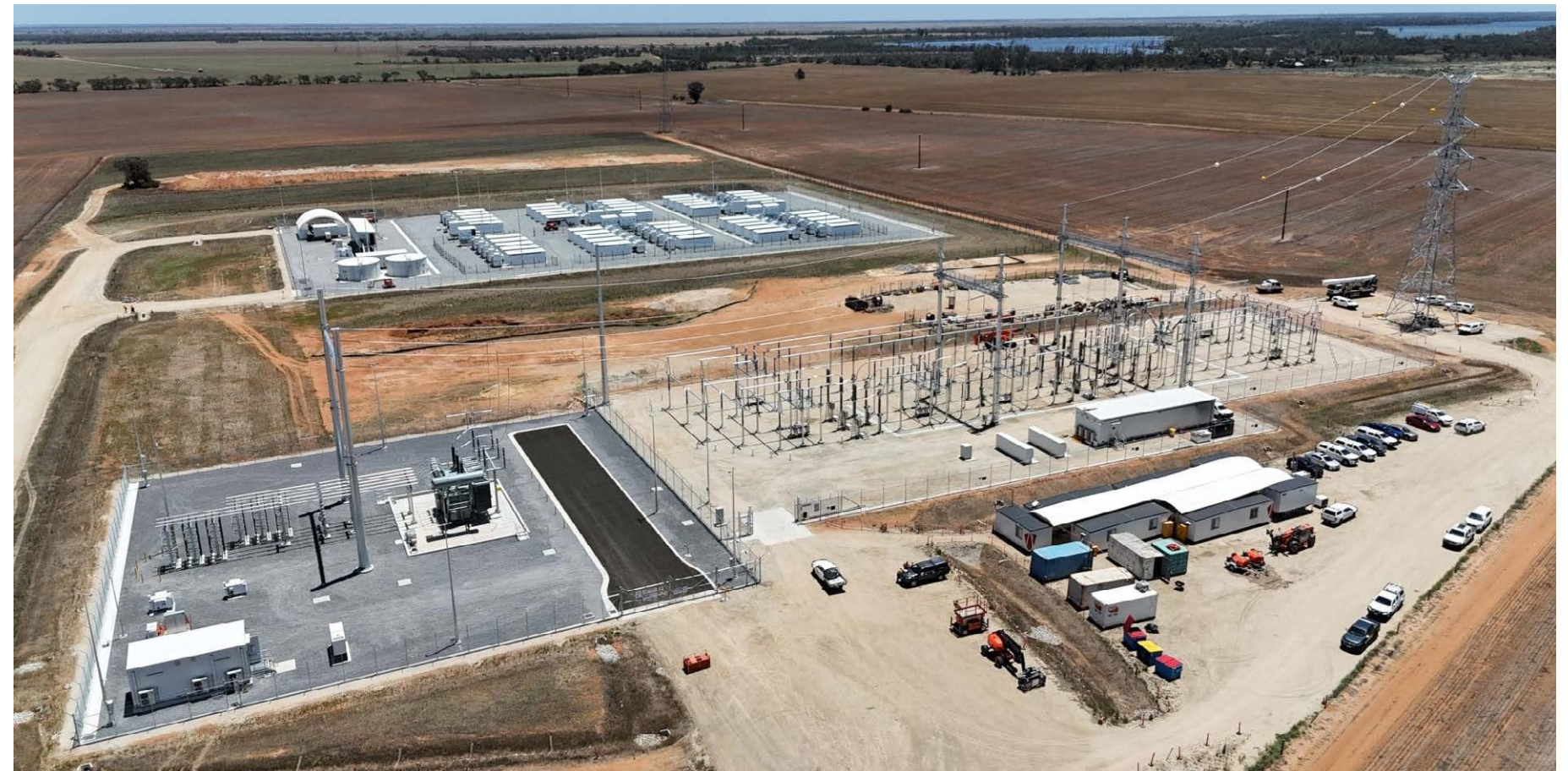
Figure 8 Example of a Terminal Station and BESS facility (Source: Potentia Energy)
