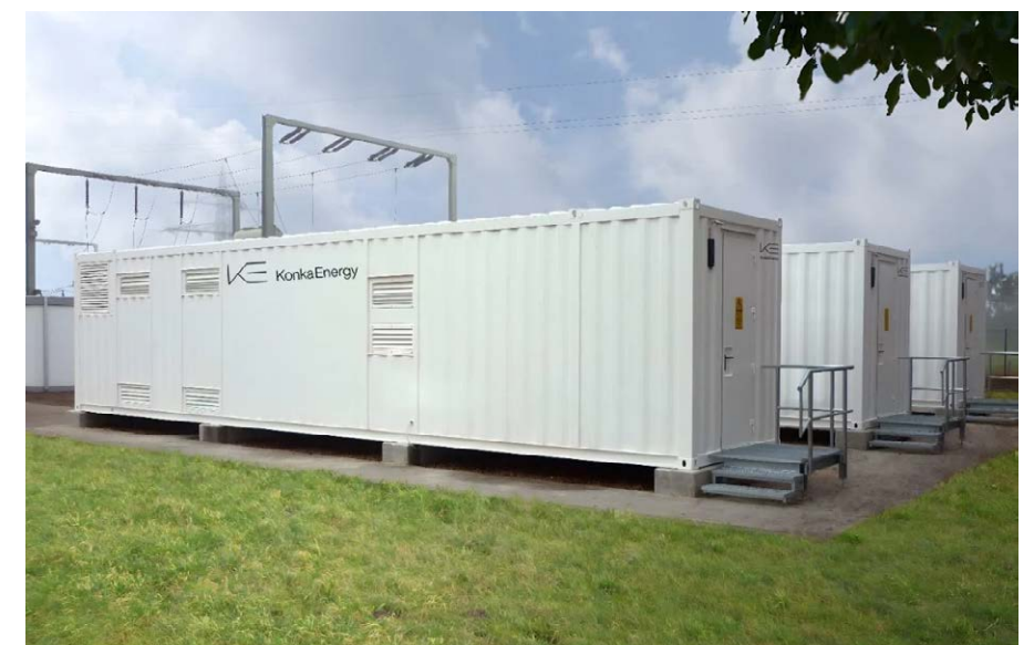
Figure 10 Indicative 40 foot BESS container (Source: Konka Energy)
