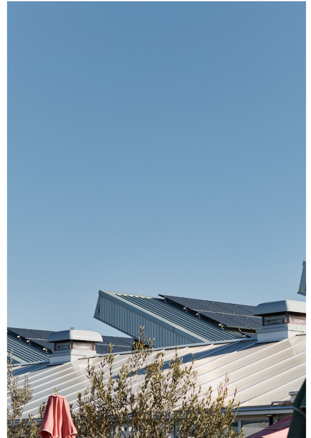
Rooftop Solar at Burwood Brickworks. Photography by Kim Landy.
