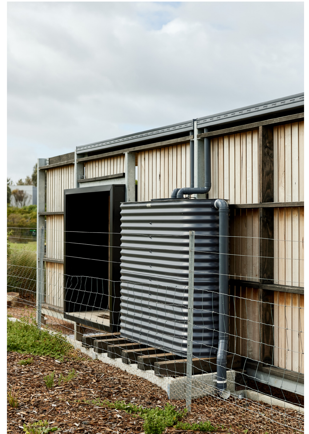
Rainwater tanks at The Cape, Cape Paterson. Photography by Kim Landy.
