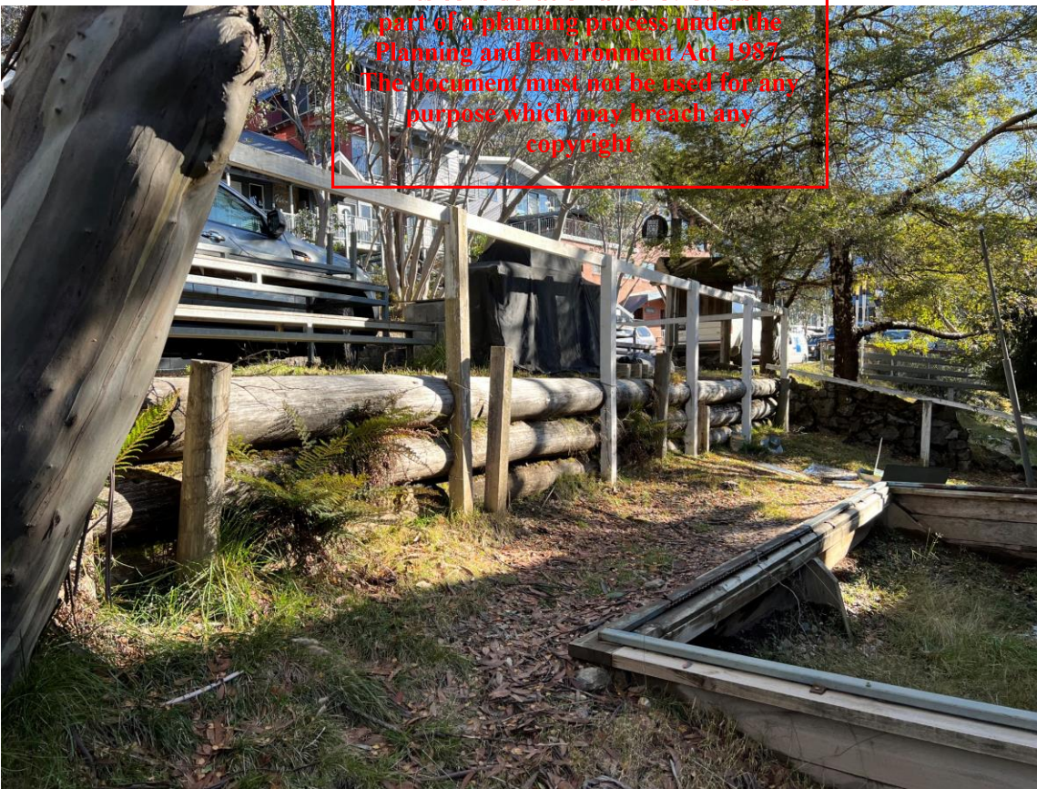
Figure 8 Log retaining wall along the southern boundary of the property. The retaining wall is situated between the front of the property and Parallel Street
