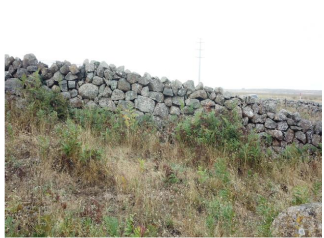
Plate 4: The East-West aligned part of DSW-1 showing poor bonding (A. Wilkinson 2020).
