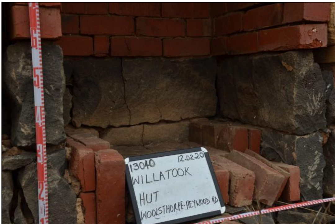
Plate 22: VHI H7321-0104 (Woolsthorpe-Heywood Road Hut 1). Detail of bricks inside chimney structure indicating replacement and/or reuse. Photo A. Wilkinson
