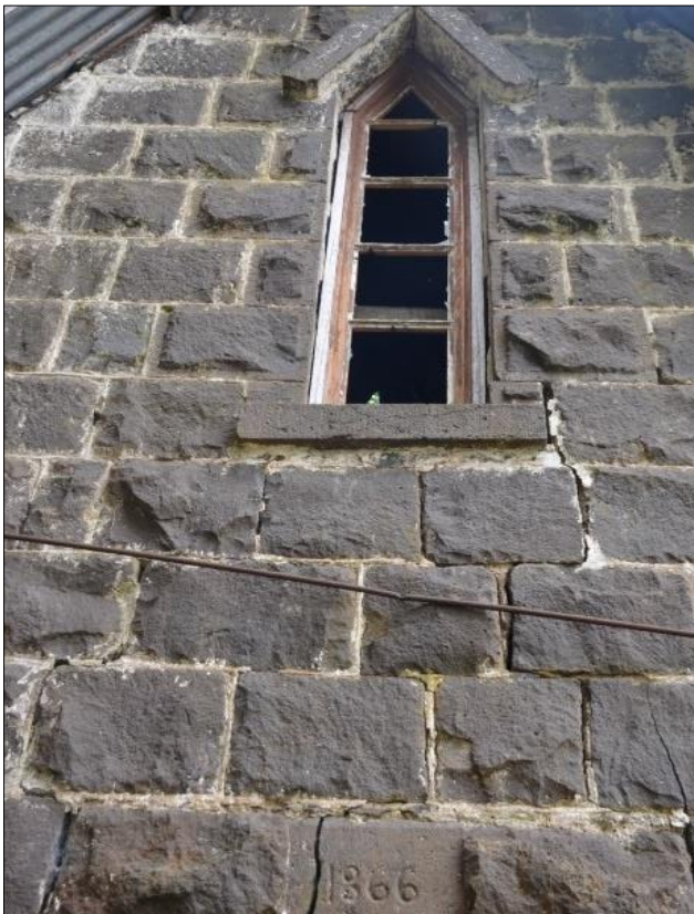
Plate 13: Detail of highlight window and stepped cracking on front of Bath House. View North. Photo A. Wilkinson
