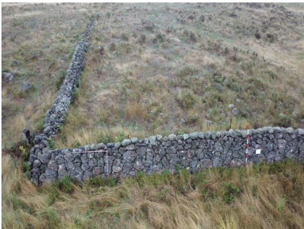
Plate 3: DSW-1 showing collapse at the corner where walls meet facing east (A. Wilkinson 2020).
