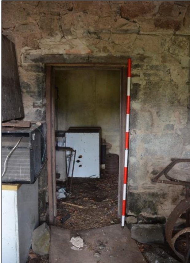
Plate 12: Internal wall showing original layout of two rooms, wooden door frame. Photo A. Wilkinson
