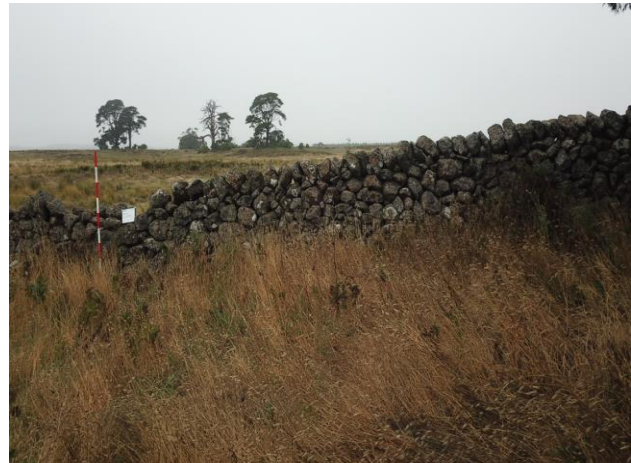
Plate 10: The middle section of DSW-2 showing collapse (A. Wilkinson 2020).
