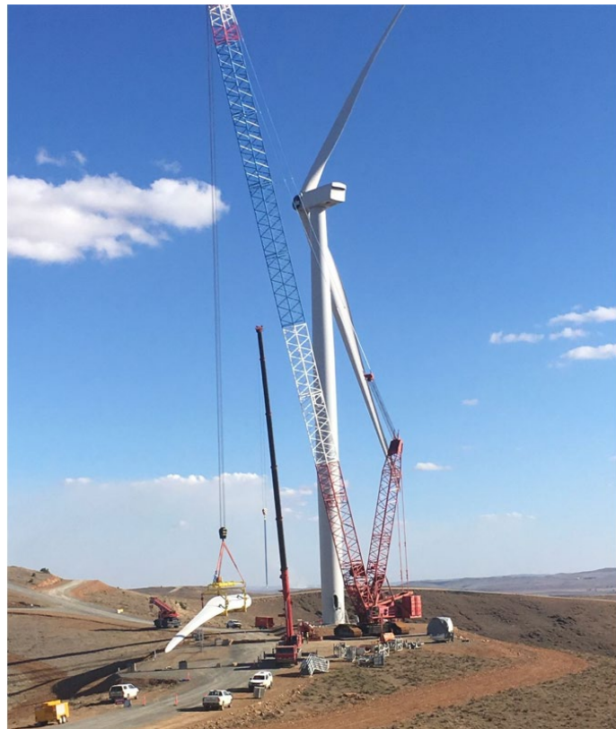
Figure 3-7 A rotor with three blades with the final blade being lifted onto a wind turbine tower
