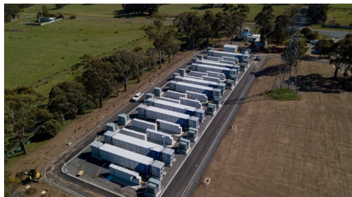
Figure 3-12 Example 30-megawatt battery system at Ballarat, Victoria
