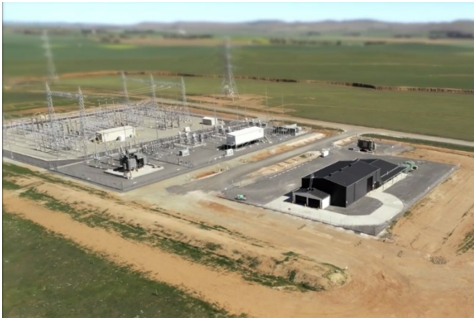
Figure 3-10 Example of wind farm substation and operations and maintenance facility
