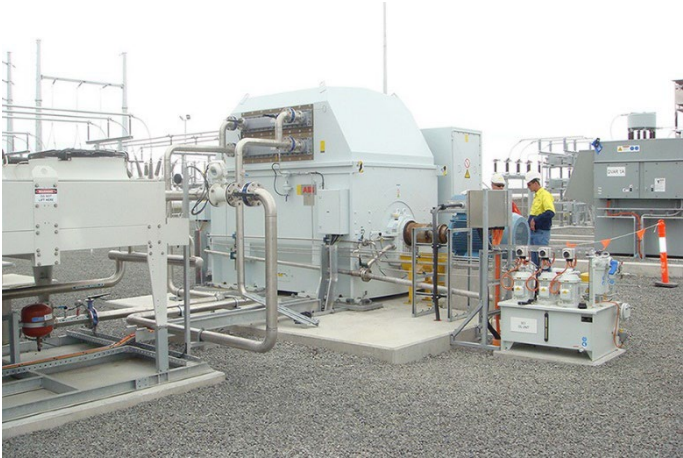
Figure 3-11 Example synchronous condenser
