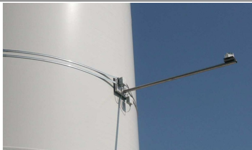
Light sensor mounted to the tower of a wind turbine
