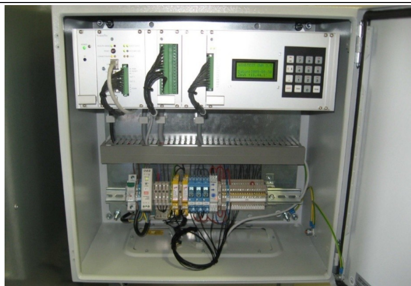
Shadow flicker module cabinet with cabling
