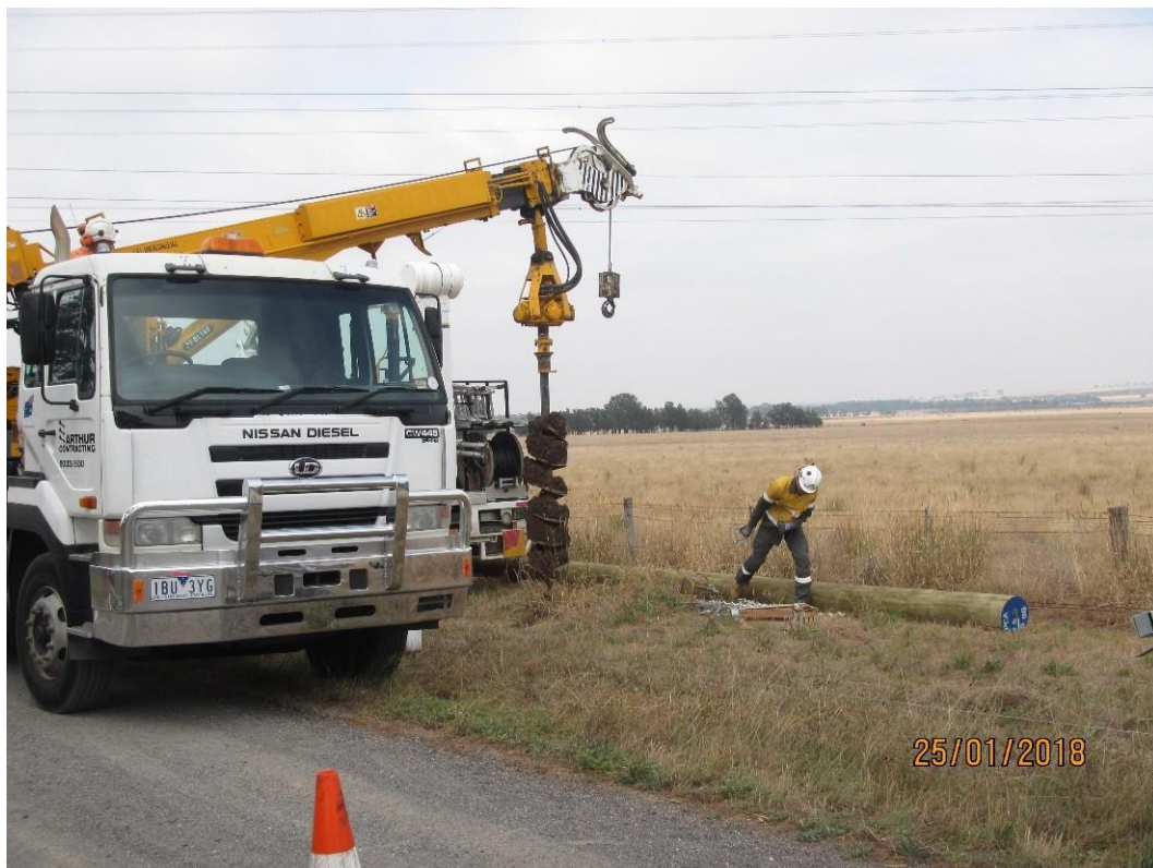
Figure 2: Example of a hole being augered via arm from truck (note in this example the roadside vegetation was deemed to be non-native, hence the truck parking slightly on the verge and the other truck in the background).
