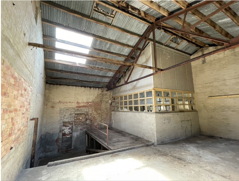
Part of the internal layout of the western bay showing timber framed glazing, ladders, and stairs etc
