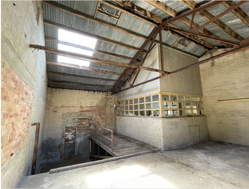
Part of the internal layout of the western bay showing timber framed glazing, ladders, and stairs etc
