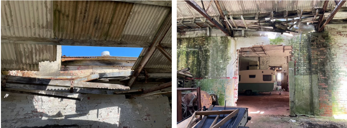
Missing sections of roof and failing sections of the central box gutter. Also note the lack of lintel to the added opening on the right.
