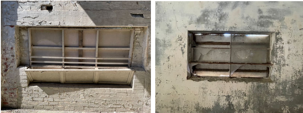
Façade windows in the east (left) and west (right) bays as viewed internally.
