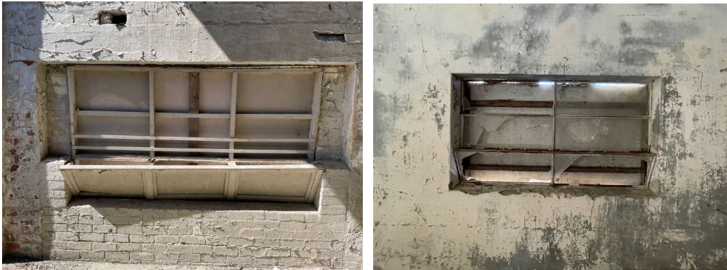
Façade windows in the east (left) and west (right) bays as viewed internally.
