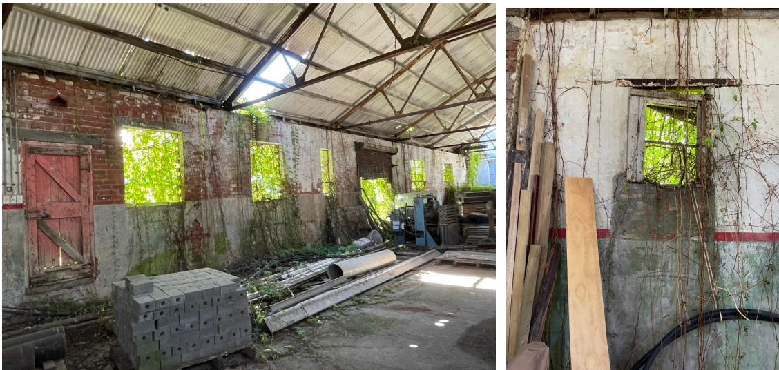
At left, Window openings along the east wall. At right, partially infilled timber window
