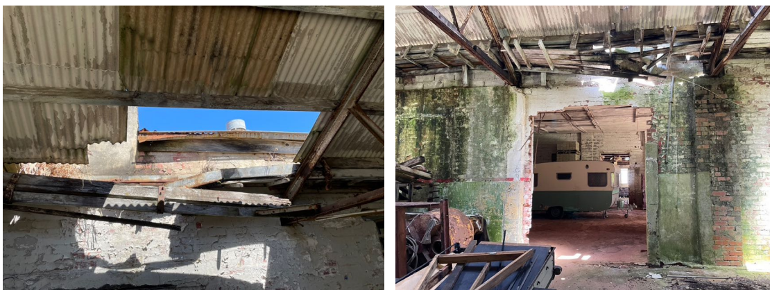
Missing sections of roof and failing sections of the central box gutter. Also note the lack of lintel to the added opening on the right.
