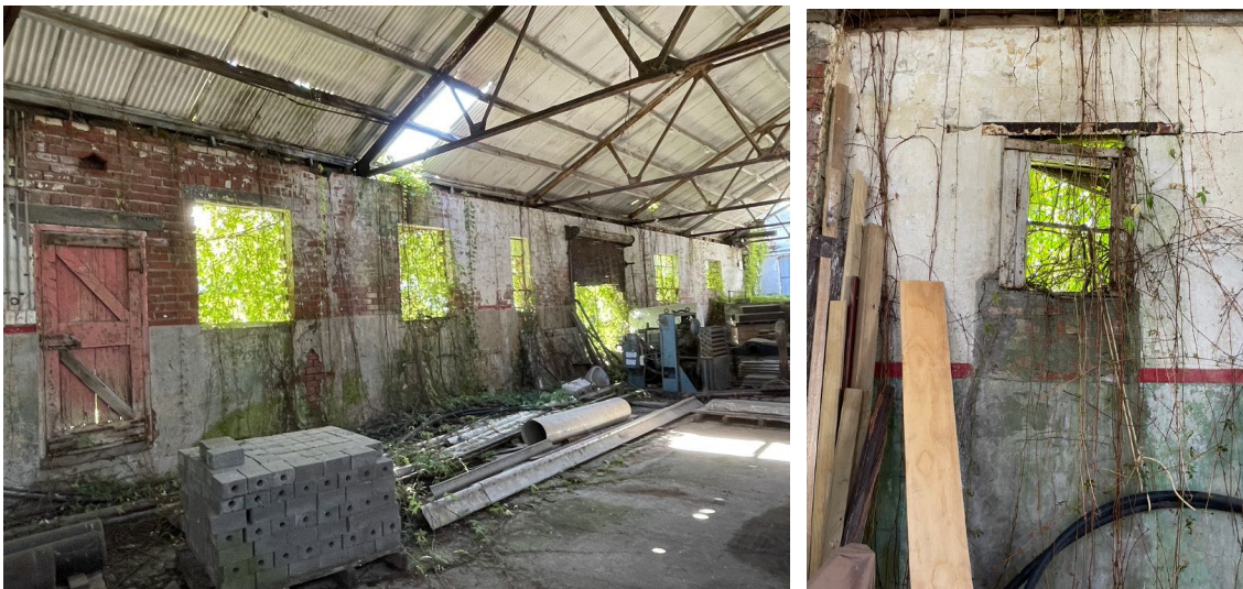
At left, Window openings along the east wall. At right, partially infilled timber window
