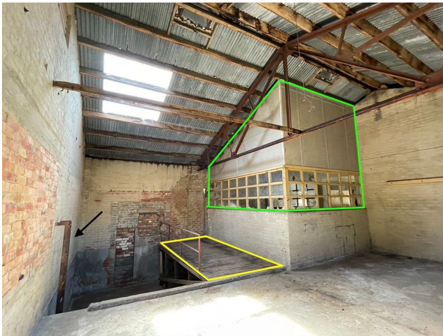
Figure 3: As shown in Figure 2, the section of original wall and glazing outlined in green will be retained as evidence of the original detailing within this space, the timber deck materials will be retained and reinstated in the floor below and the ladder at left will be retained.
