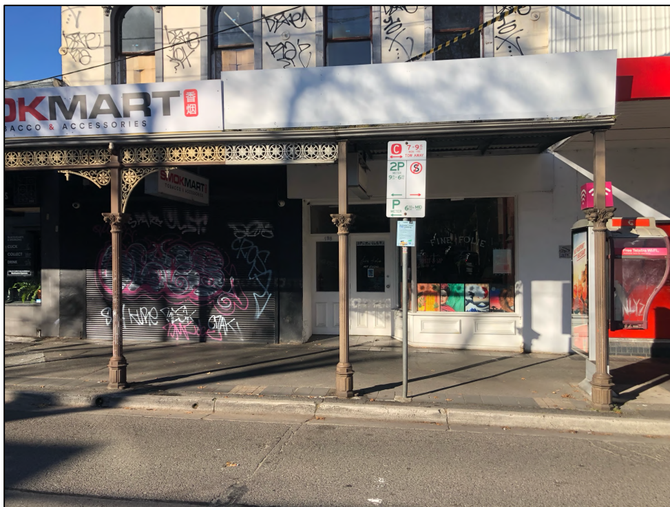
Figure 9 The existing verandah appears to have been reconstructed in relatively recent times and is incomplete.
