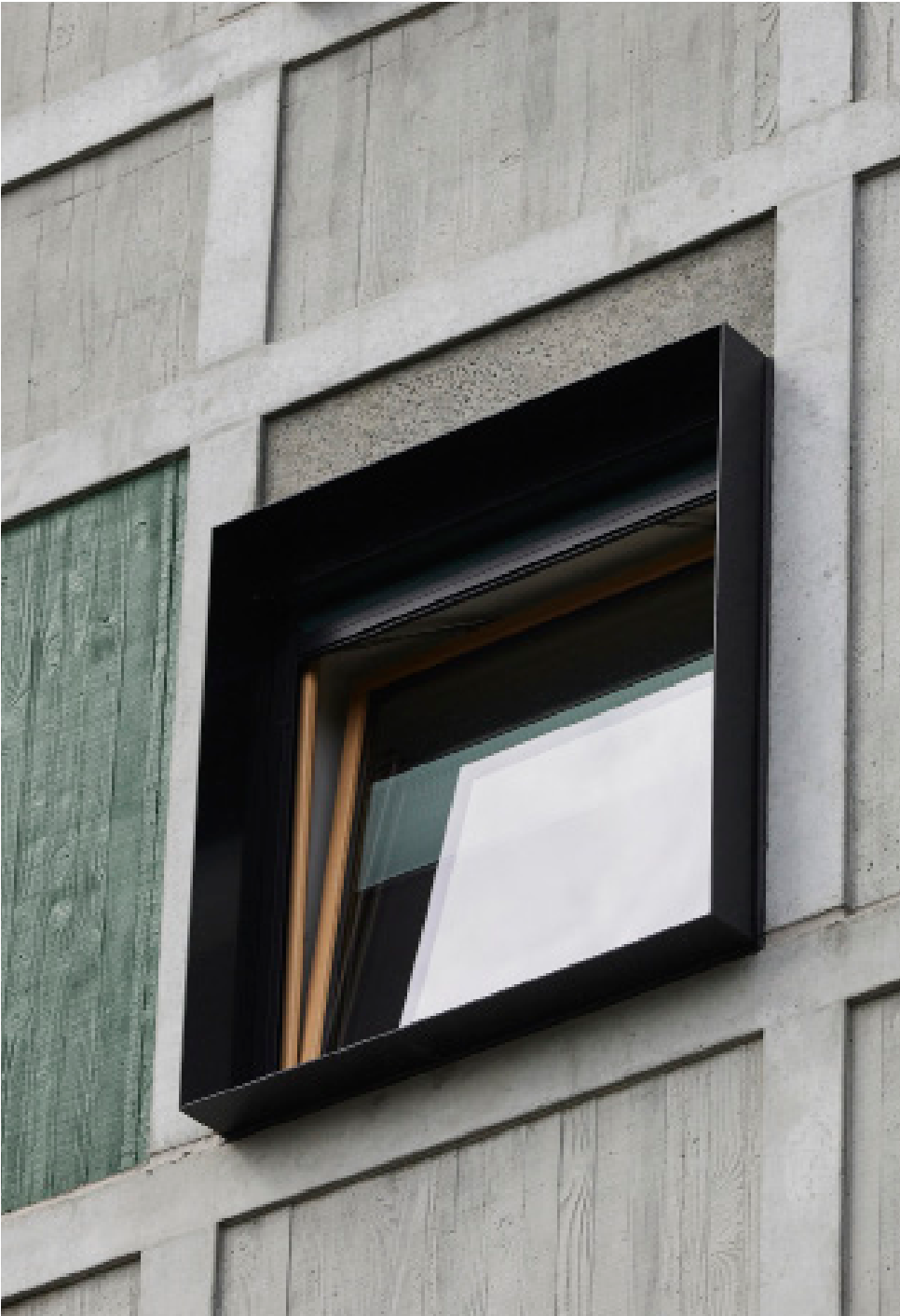
External operable blinds. Photography by Kim Landy.
