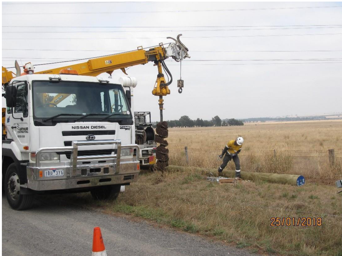
Figure 2. Example of a hole being augured via arm from truck (note in this example the roadside vegetation was deemed to be non-native, hence the truck parking slightly on the verge and the other truck in the background)
