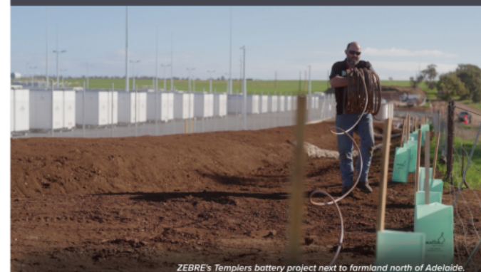
ZEBRE's Templers battery project next to farmland north of Adelaide.
