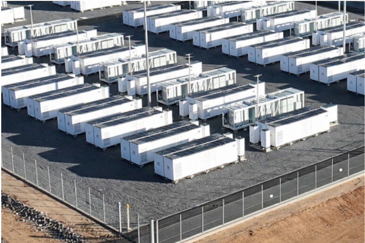
Figure 1-2 Example of battery storage units
