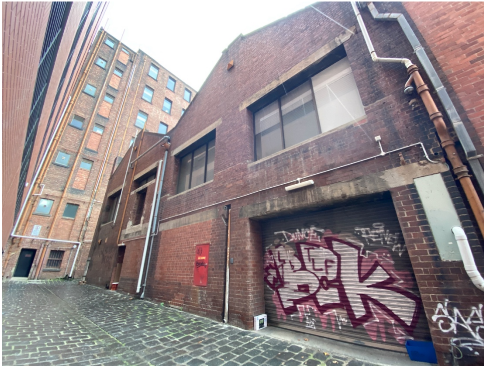
Figure 5: View of the rear (north) elevation to McDougall Lane. Note the extent of alterations. Source: Trethowan Architecture.
