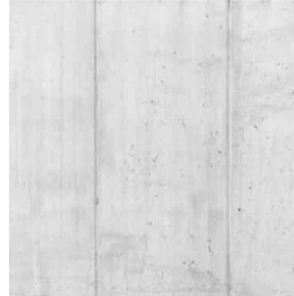
CODE: C-02 DESCRIPTION: ARCHITECTURAL CONCRETE MATERIAL: PRE-CAST CONCRETE PANELS FINISH: OFF-FORM FINISH CLASS 1 COLOUR: WHITE BRIGHTONLITE CEMENT (INTEGRAL OXIDE COLOUR)
