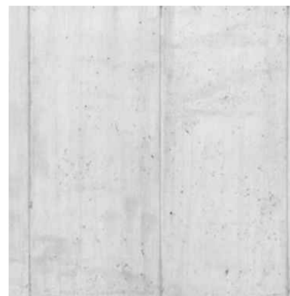
CODE: C-03 DESCRIPTION: ARCHITECTURAL CONCRETE MATERIAL: INSITU CONCRETE COLUMNS & SLABS FINISH: OFF-FORM FINISH CLASS 2 COLOUR: WHITE BRIGHTONLITE CEMENT (INTEGRAL OXIDE COLOUR)
