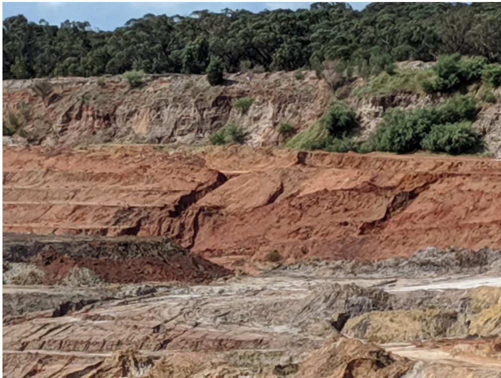
Figure 15 Example of Erosion of Exposed Sand Batters at Nearby Quarry
